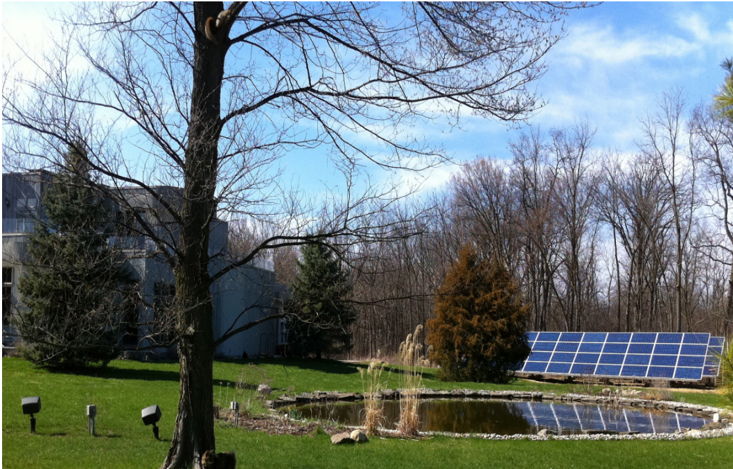
2 arrays with each 44 MAGE POWERTEC Plus 225/6 panels are powering the 19.8 kW installation near Ann Arbor, MI. © SUR Energy LLC.
