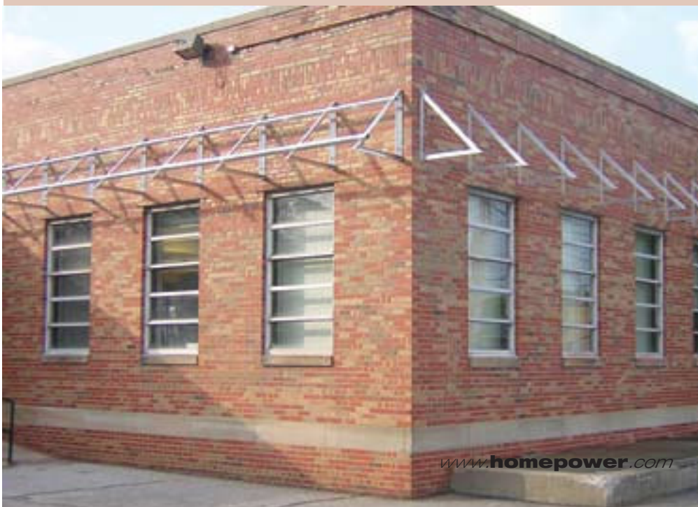
Custom-made mounting brackets provide a stable platform for the PV arrays.
