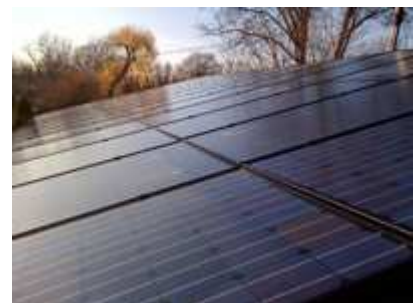
8 kW Electric System (Largest residential PV systems in Wayne County) Garden City, MI
