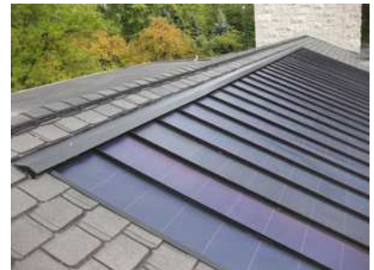
3.7 kW Laminated Electric System Governor's Residence Lansing, MI
